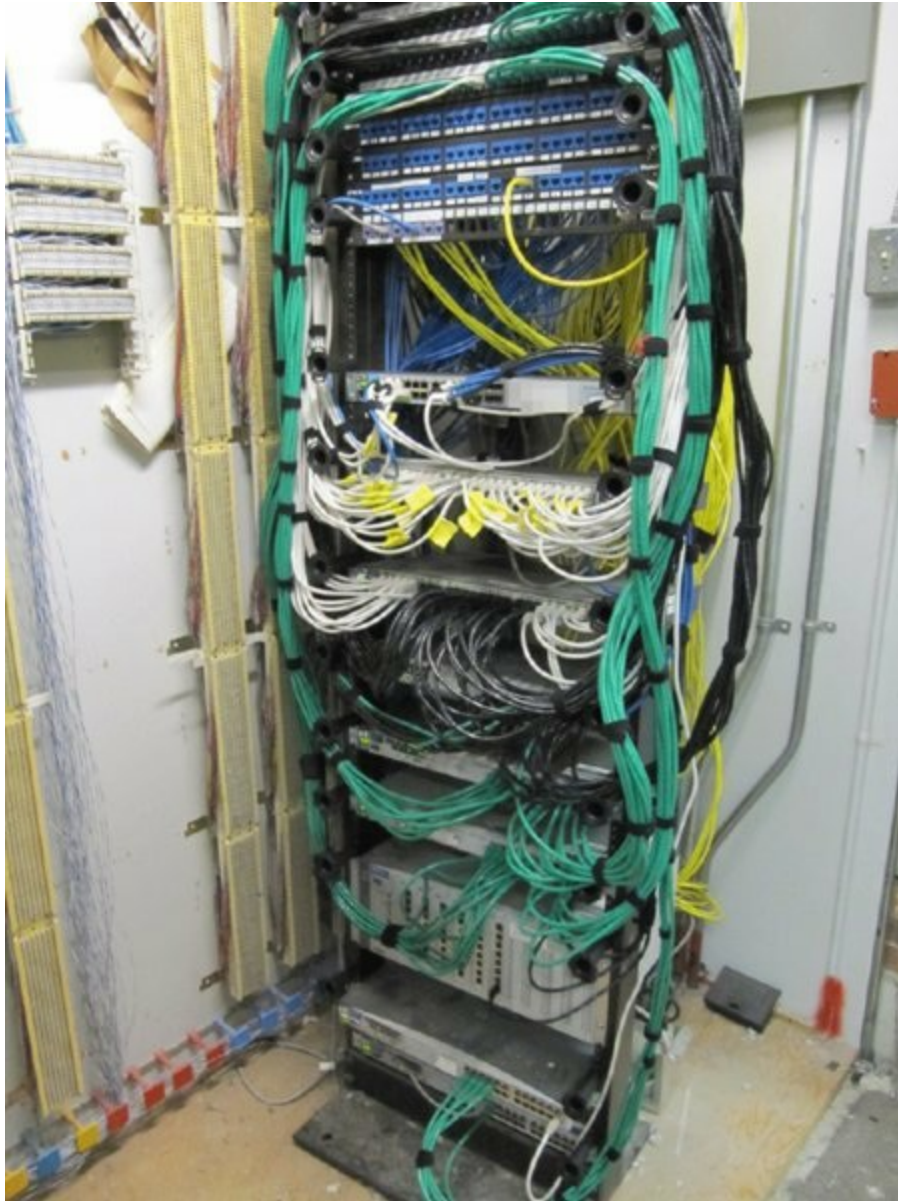
Figure 10.1 A typical wiring closet
